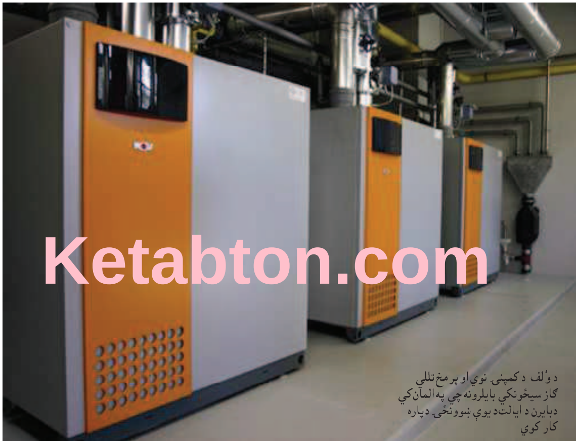
Wolf MGK gas condensing commercial boiler with cascade control Hot trio for the secondary school in Au, Hallertau (Bavaria - Germany)
